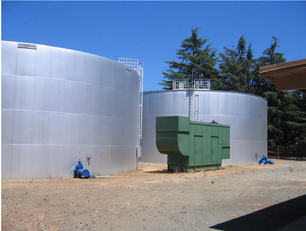
Figure 2-26. Hamilton Tanks (#2 foreground, #1 background) and Emergency Generator, showing 10" Outlet Pipes
