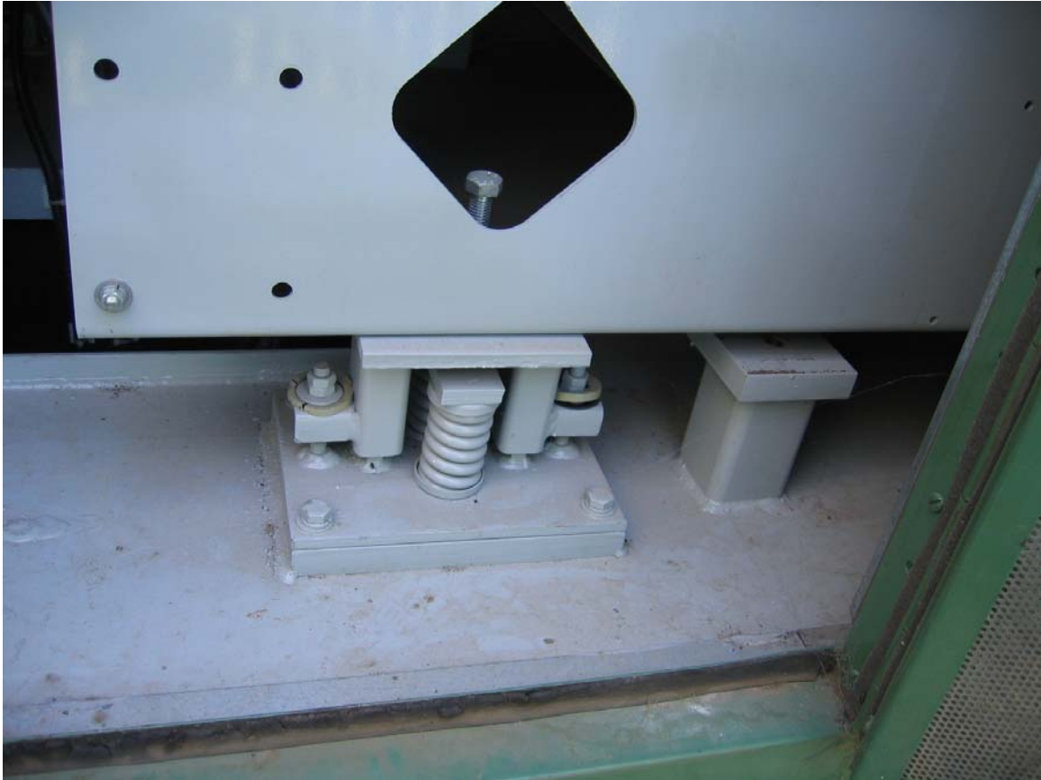
Figure 2-63. Raynor Well – Emergency Generator Isolator Mounts
