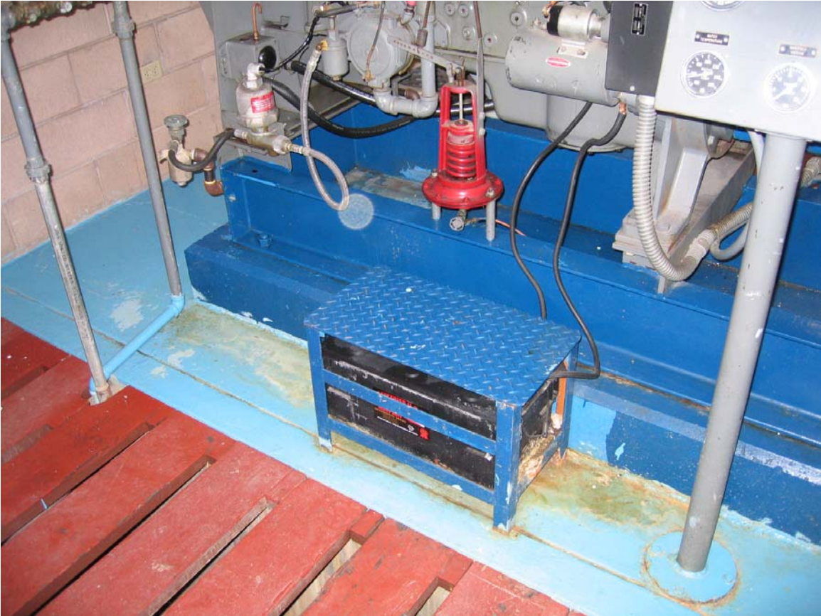
Figure 2-24. Wright Avenue Pump Station – Start-Up Battery for Backup Engine
