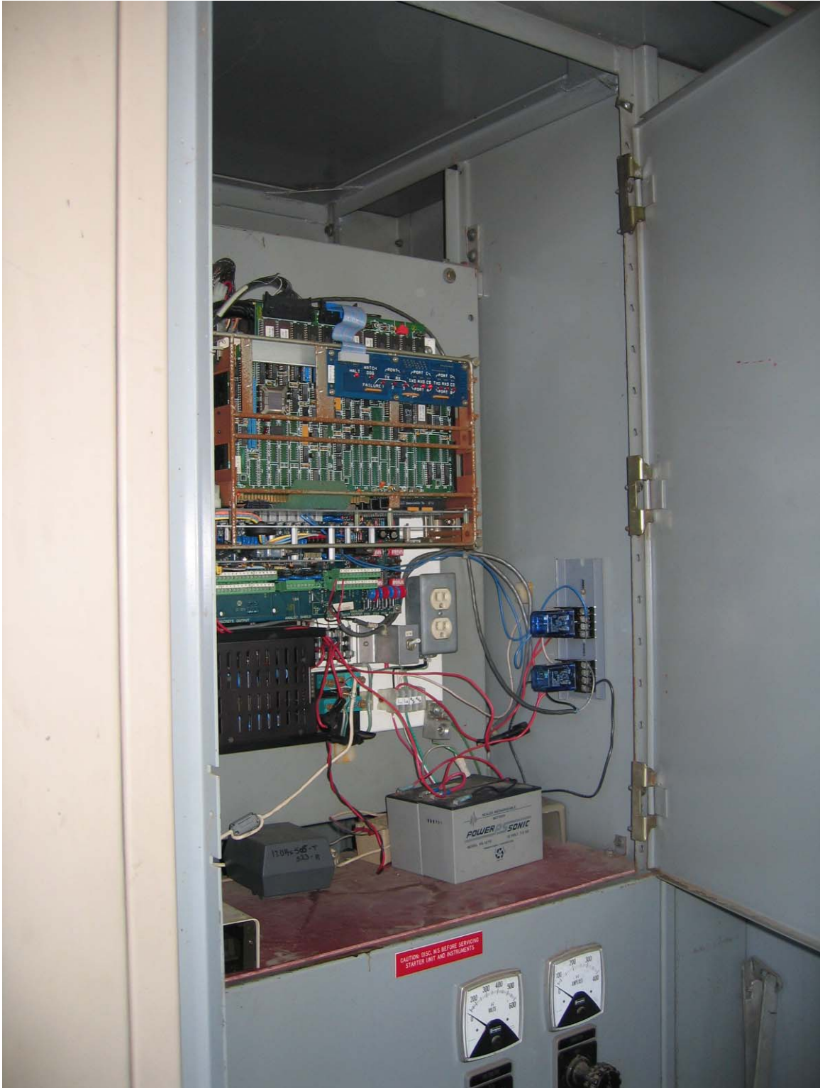
Figure 2-61. Raynor Well – SCADA Batteries
