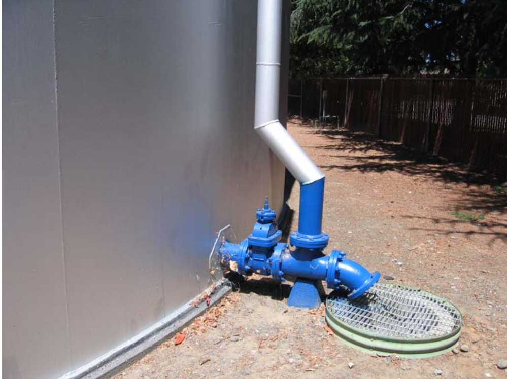
Figure 2-33. Hamilton Tank #3 Overflow and Drain Pipe
