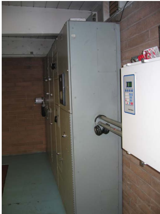
Figure 2-17. Mary Carson Pump Station – Electrical Cabinet
