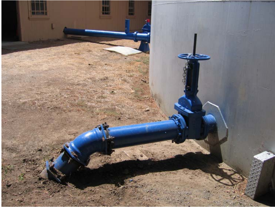
Figure 2-42. Central #2 Inlet-Outlet (Restrained Joints) and 10" Outlet pipe to pump station (background)
