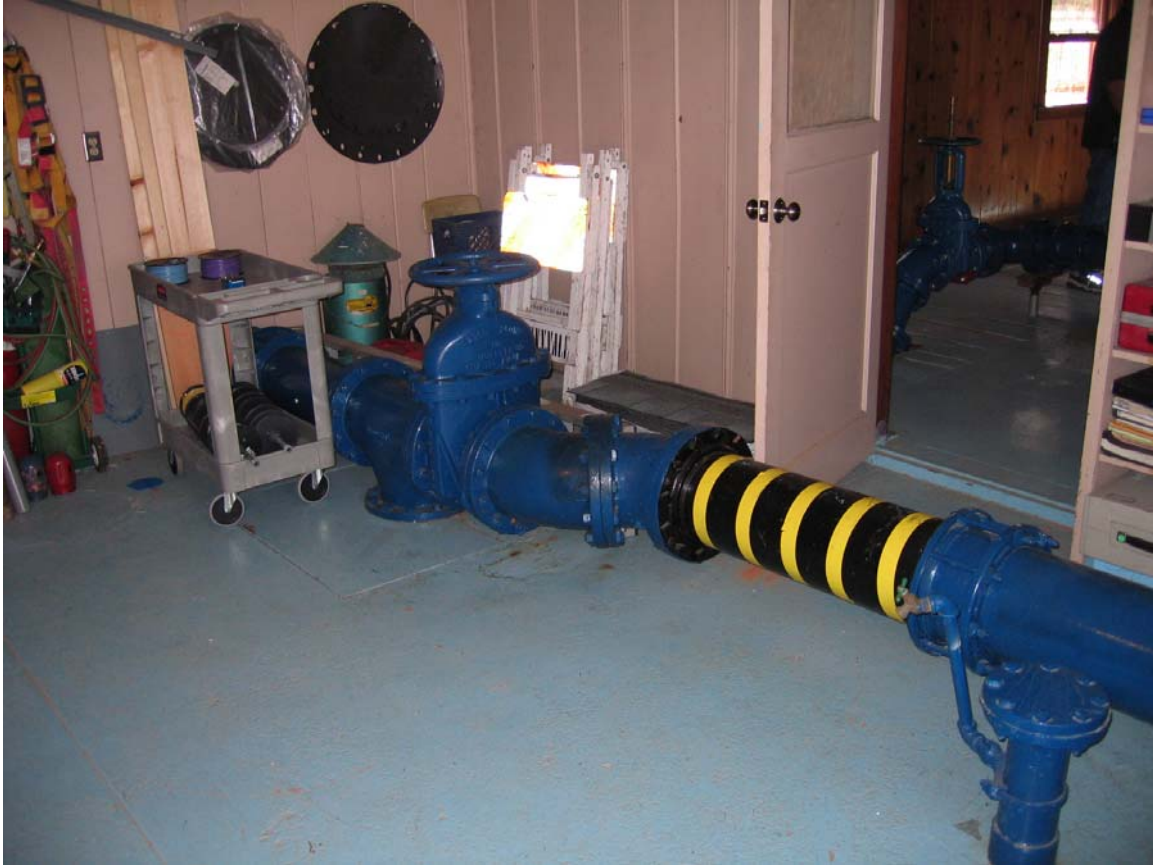
Figure 2-46. Central Pump Station Suction Pipe Inside Building
