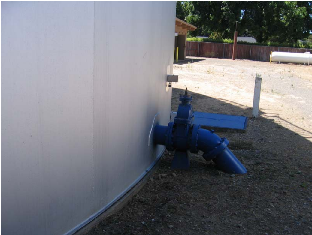
Figure 2-29. Hamilton Tank #3 10" Outlet Pipe
