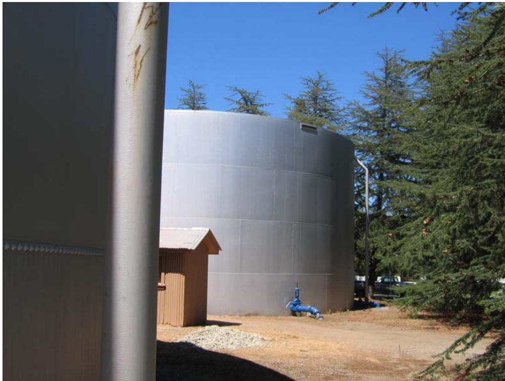
Figure 2-41. Tank #2 (background) Inlet-Outlet and Overflow/Drain
