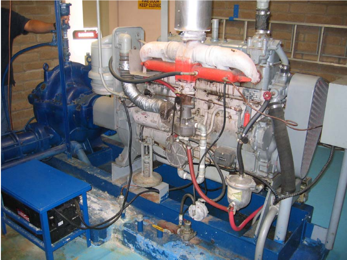
Figure 2-37. Engine and Start-Up Battery for Hamilton
