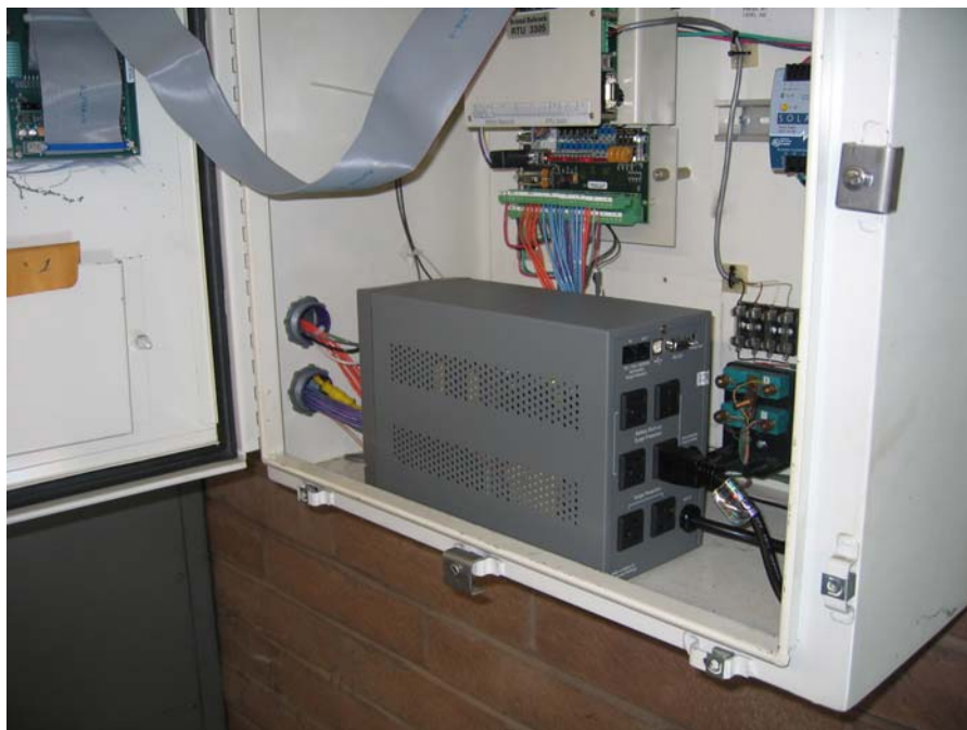
Figure 2-19. Mary Carson Pump Station –SCADA Cabinet and Battery
