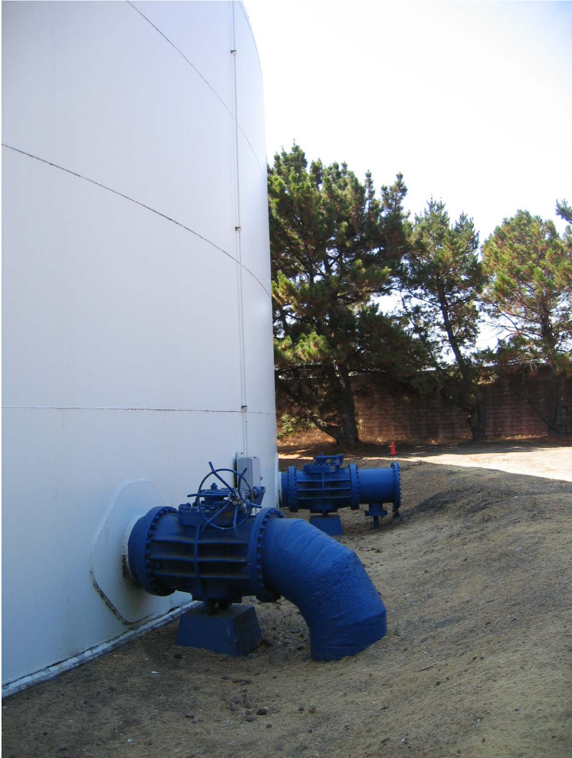
Figure 2-20. Wright Avenue Tank 1 – 30" Outlet Pipe (Foreground) and 30" Spare Outlet (Background)
