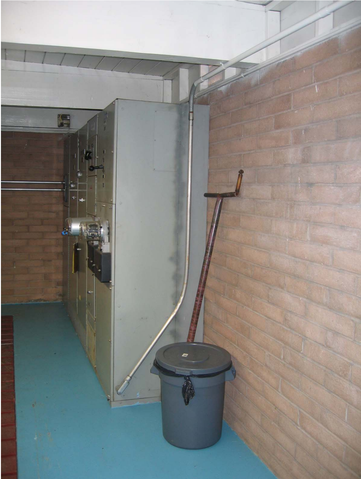
Figure 2-53. Wolfe-Evelyn Pump Station Electrical Controls
