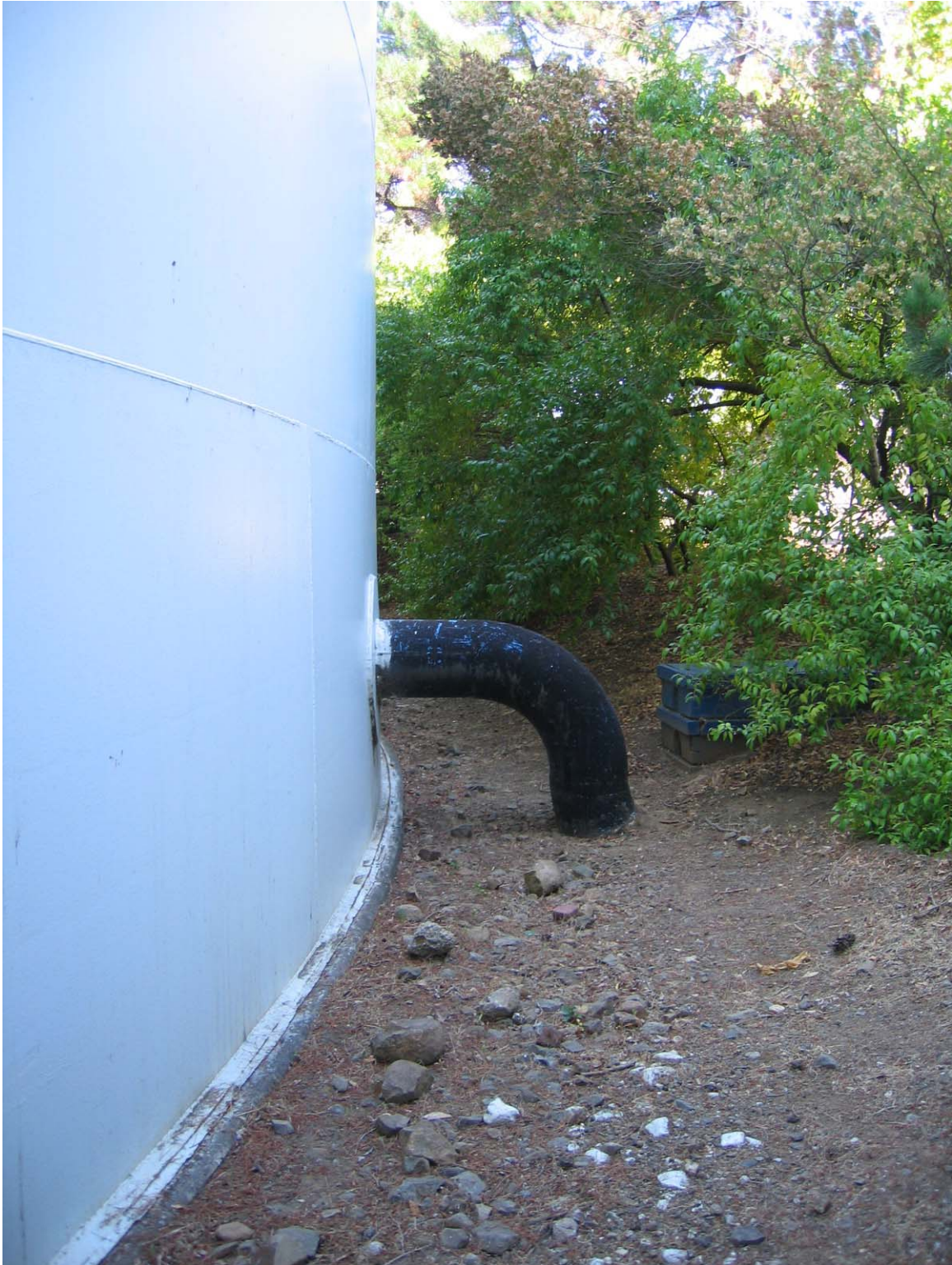
Figure 2-22. Wright Avenue Tank 2 – Overflow Pipe
