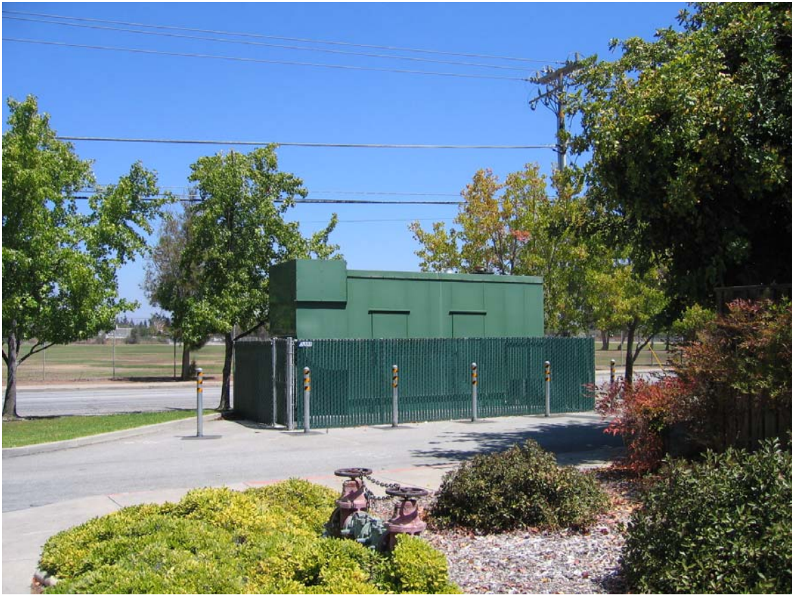
Figure 2-62. Raynor Well – Emergency Generator
