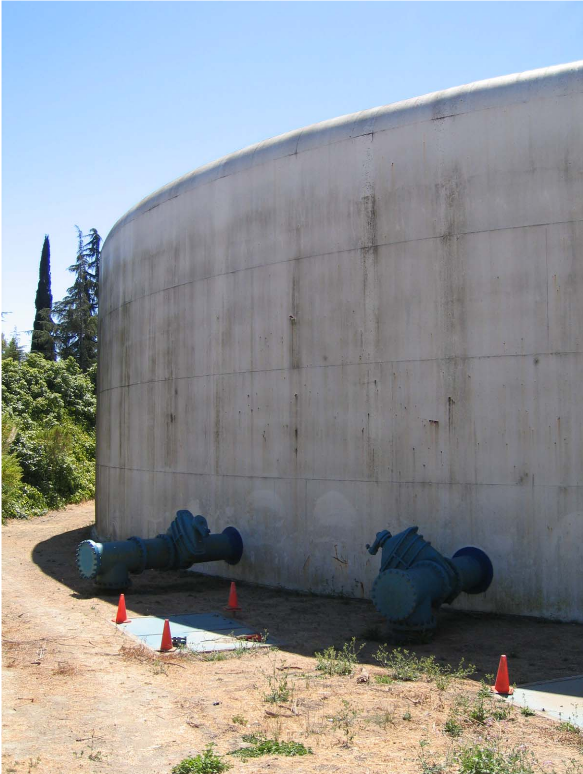
Figure 2-50. Wolfe-Evelyn Tank –24" Inlet (foreground) and 24" Outlet (background) Pipes
