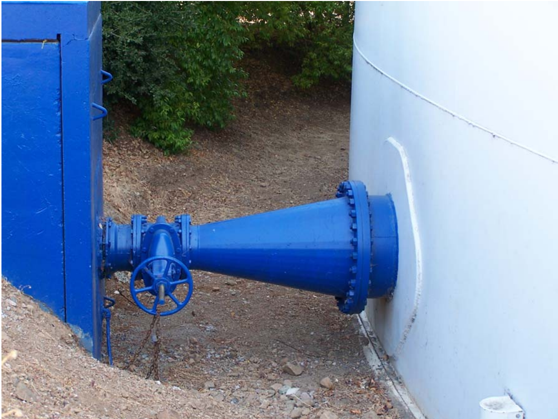
Figure 2-21. Wright Avenue Tank 2 – 30" Inlet Pipe with Reducer to Vault
