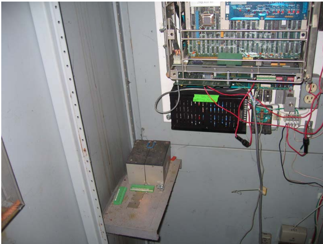
Figure 2-59. Ortega Well – SCADA Batteries
