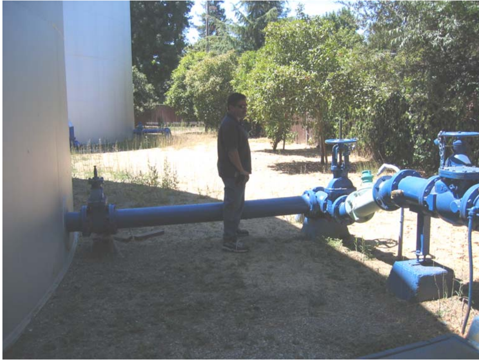
Figure 2-30. Hamilton Tank #1 8" Inlet Pipe from Well #2
