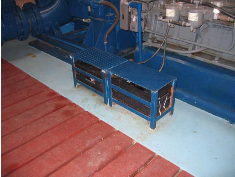
Figure 2-18. Mary Carson Pump Station – Start-Up Batteries
