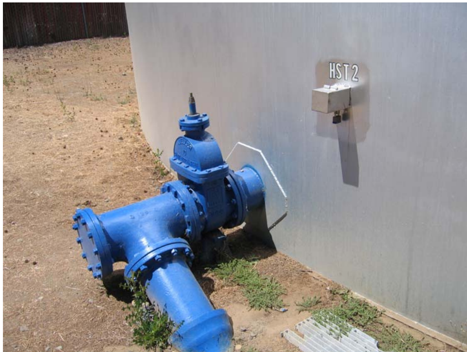
Figure 2-31. Hamilton Tank #2 10" Outlet Pipe to Pump Station
