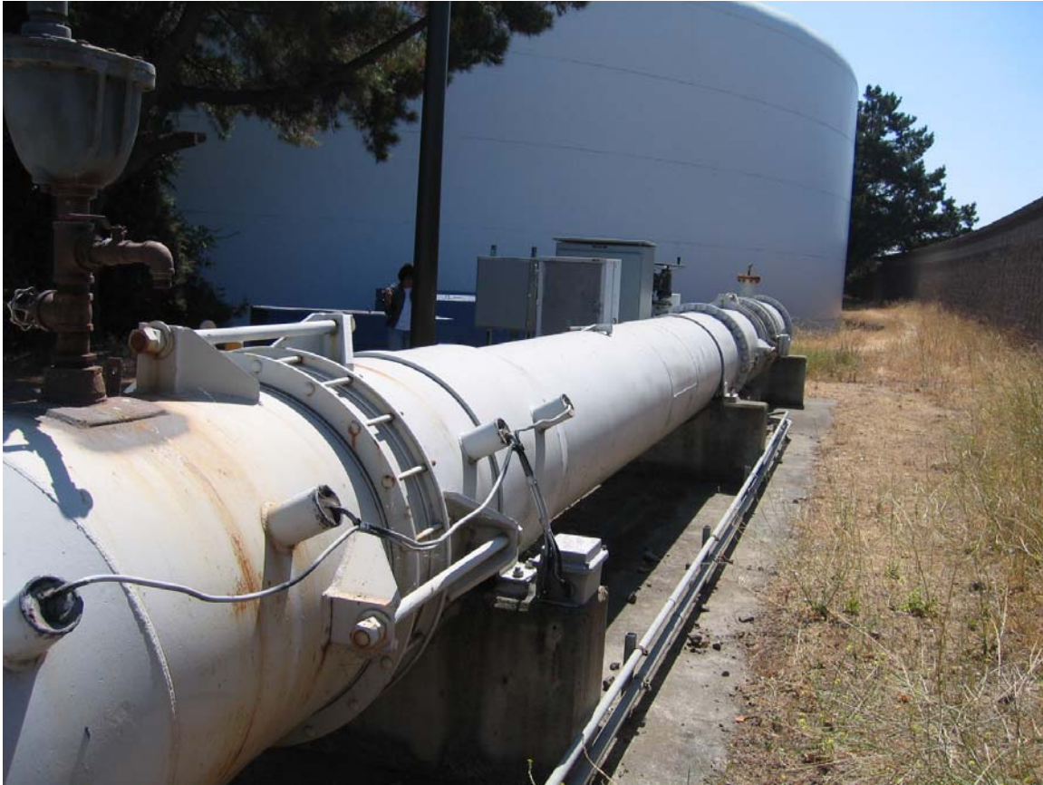
Figure 2-25. SCVWD Turnout Pipeline at Wright Avenue (Tank 2 in background)
