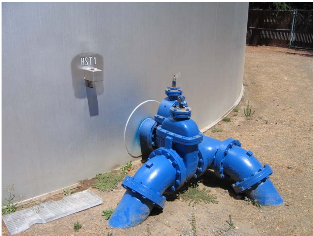
Figure 2-27. Hamilton Tank #1 10" Outlet Pipe
