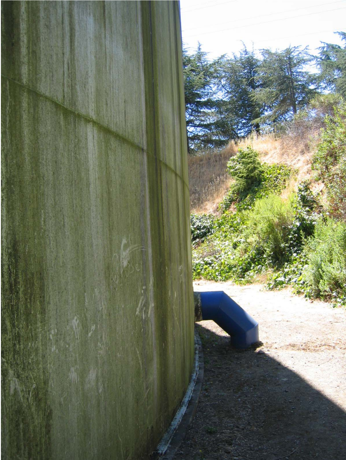
Figure 2-51. Wolfe-Evelyn Tank 16" Overflow Pipe
