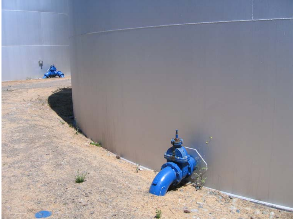
Figure 2-28. Hamilton Tank #3 (foreground) 8" Inlet Pipe
