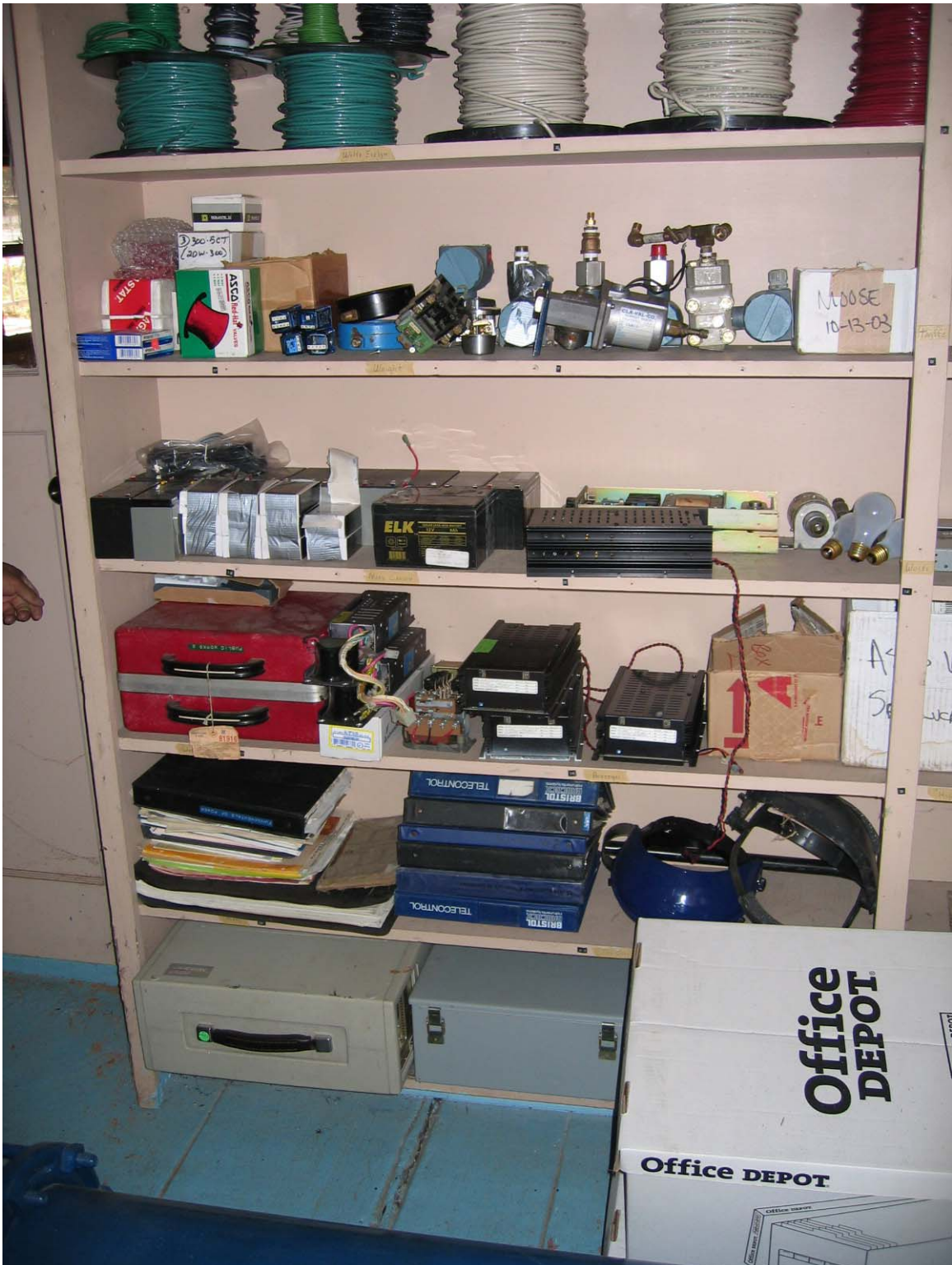
Figure 2-48. Central Pump Station Storage Shelves
