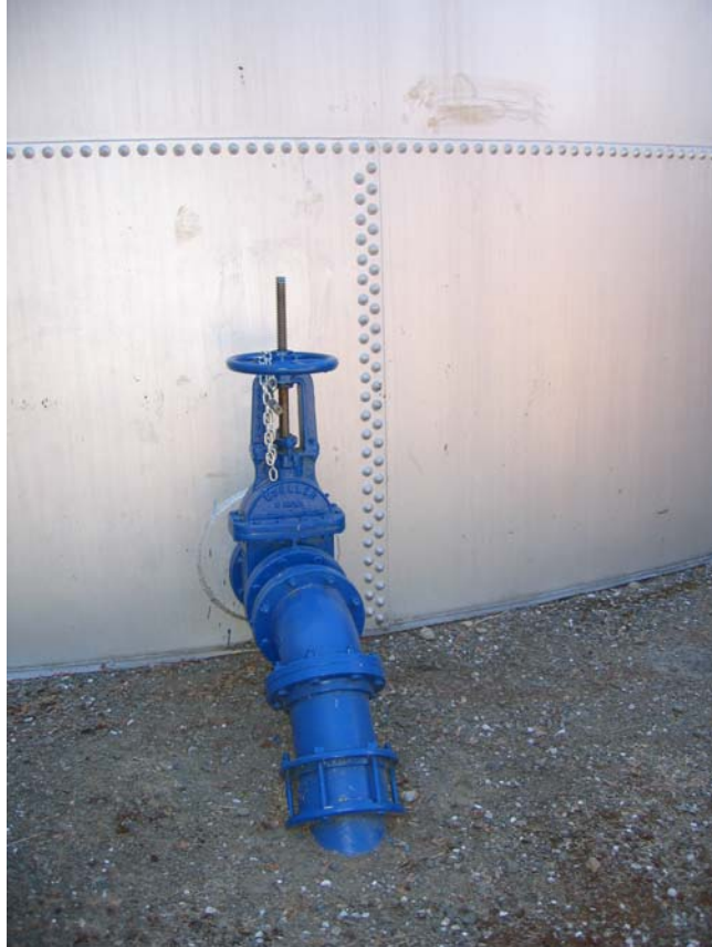
Figure 2-38. Tank #1 8" Inlet Pipe
