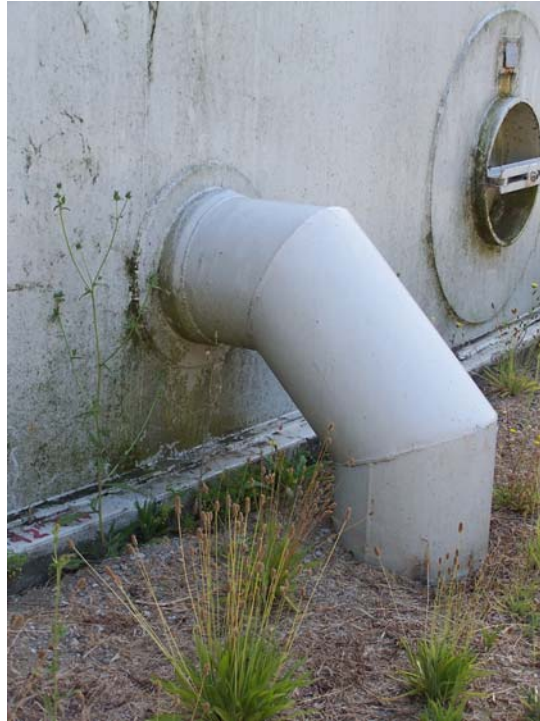
Figure 2-10. Mary Carson Tank 1 Overflow
