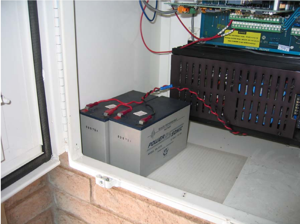
Figure 2-57. Serra Well SCADA Batteries
