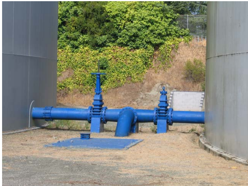
Figure 2-12. Mary Carson Tank 2 (left) and Tank 1 (right) and Outlet Pipes
