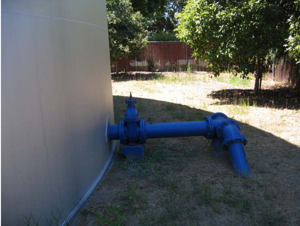
Figure 2-32. Hamilton Tank #2 8" Inlet Pipe from Well
