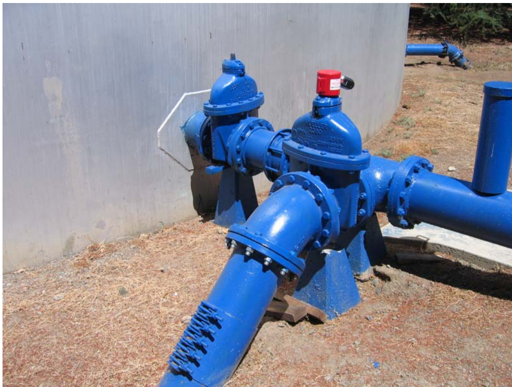
Figure 2-43. Central #2 10" Outlet Pipe to Pump Station (right) and to System (going underground)
