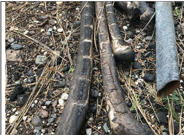
Plastic pipes can be damaged by heat and fire contact. Andrew Whelton, Purdue University
