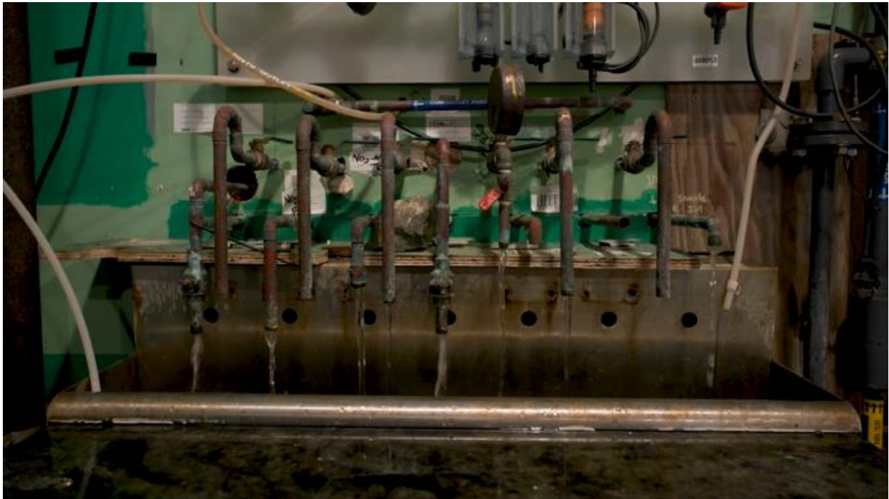
Water flows from a series of faucets in the control station at the Sunset Reservoir site | Jesse Rogala
