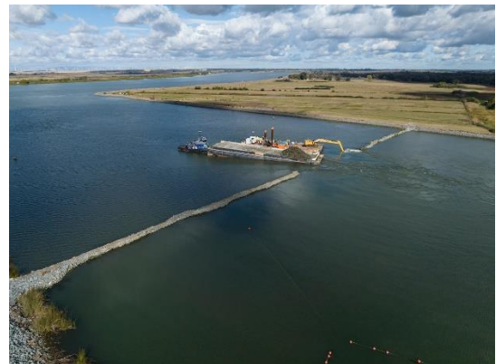
Construction crews remove Emergency Drought Salinity Barrier on the West False River near Oakley in the Sacramento-San Joaquin Delta. The rock barrier was placed to help deter the tidal incursion of saltwater from San Francisco Bay into the central Delta. Photo taken Nov. 2, 2022.
