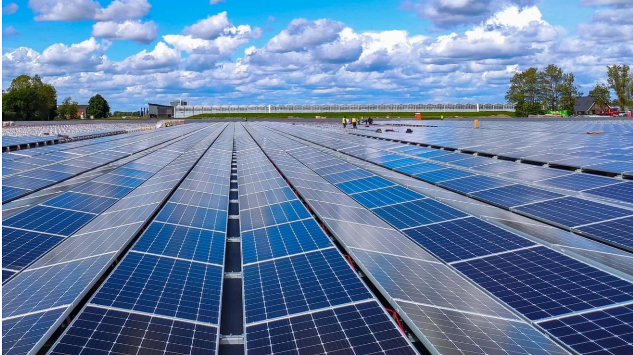
A vast solar panel array under a blue sky with clouds and workers in the background. Photo Credit: iStock
