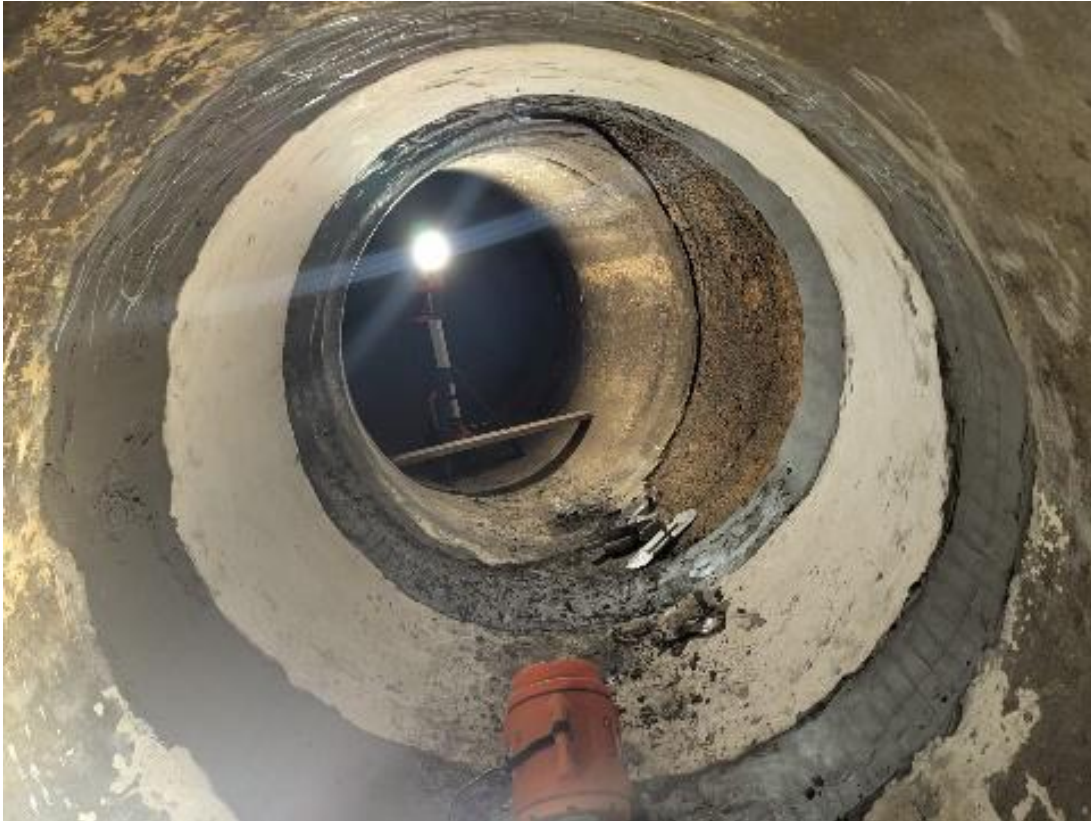
The inside of the 40-inch-long pipe spool with completion of the cement mortar lining.
