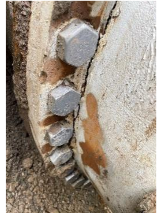
Valve failure due to water hammer
