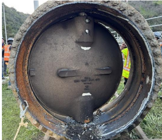
Valve position post- inspection
