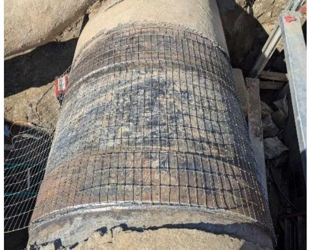
The outside of the 40-inch -long pipe spool that would later be coated with cement mortar.
