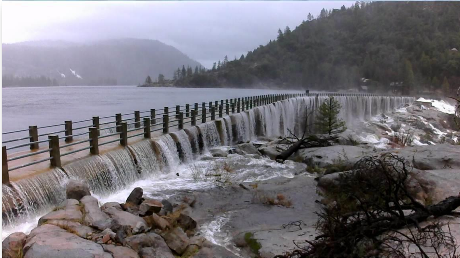
Lake Eleanor Overtopping/SFPUC, January 2017
