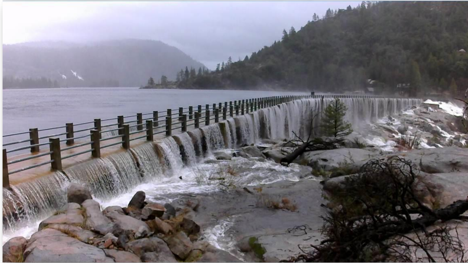
Lake Eleanor Overtopping/SFPUC, January 2017
